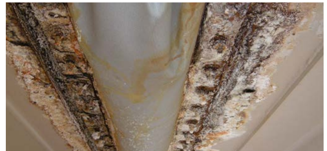
Failed stack inlet expansion joint due to corrosion
